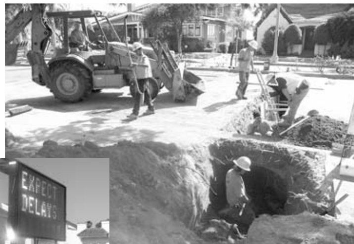
John Wood/Daily Press Above: A construction crew tends to a sewage line under Fourth Street on Tuesday afternoon. Parts of Fourth Street have been closed since Feb. 9 so the city can repave and complete work on water mains, curbs, sidewalks, the median, landscaping, crosswalks and signs. Below: Residents will have to wait longer through the summer, as work is expected to be completed by Sept. 30.
